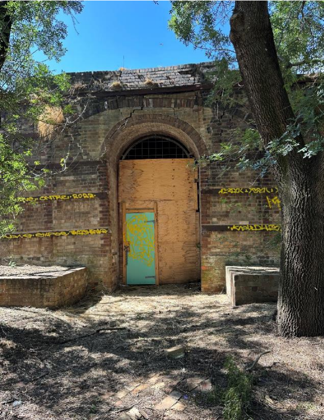
Figure 6: Entrance façade to Down Draught 2 showing the dilapidated state of the building
